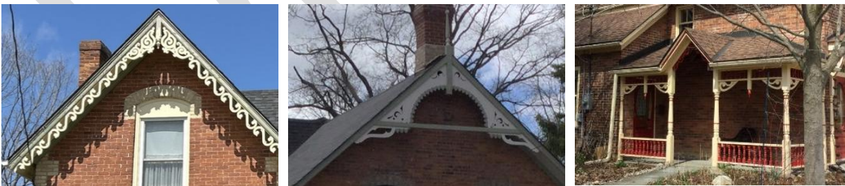
Photo 9 Examples of woodwork in the HCD including bargeboard (left and centre), window surrounds (left), and porch detailing (right)
