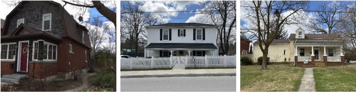
Photo 8 Examples of wood shingles (left), stucco (centre), and vinyl siding (right) in the HCD
